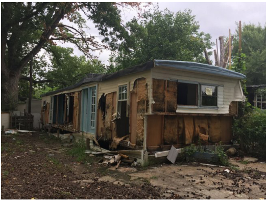
A condemned home in Rudd's
