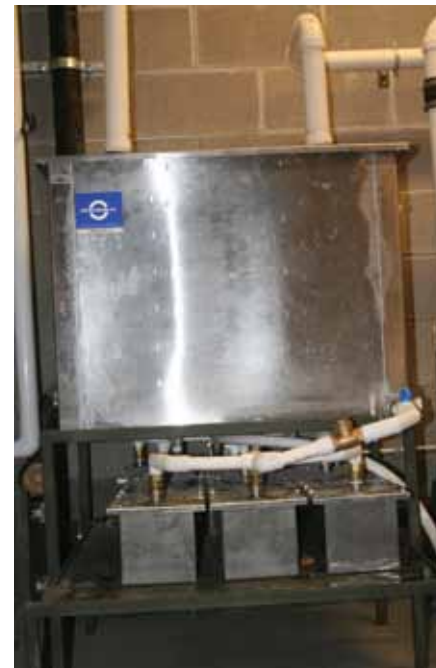
The largest of the three newly installed amalgam separators resides on the ground floor of the Perkinson Building. This unit collects amalgam waste from the Douglas and Graduate Periodontic Clinics.
