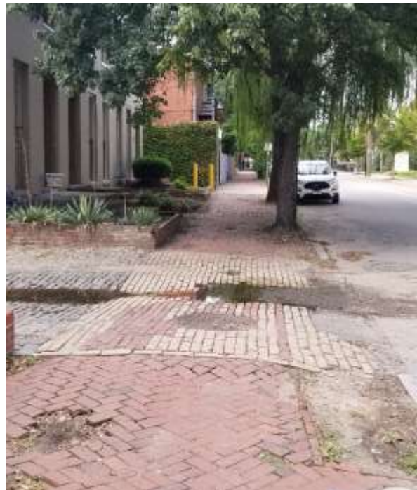
Figure 8: Harrison Street Streetscape Issues Across from VCU Campus
