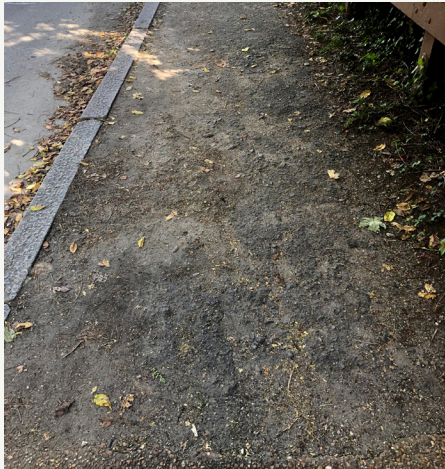
Figure 13 | Eastbound, uneven sidewalk conditions across from Belle Isle Parking Lot
