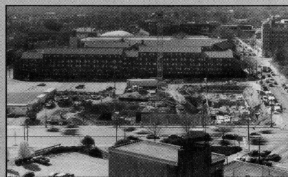
The first facilities, pictured during construction in the spring semester, in the School of Engineering complex will open for fall semester 1998.
