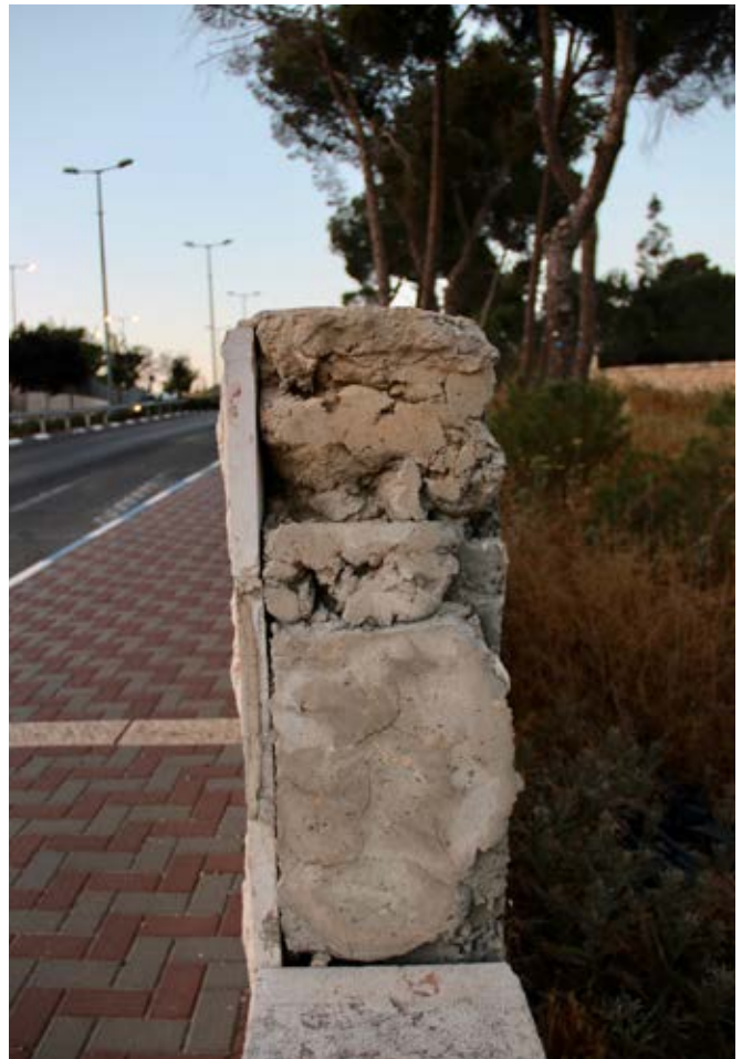
Figure 8. Crumbling of the Dastor Stone
