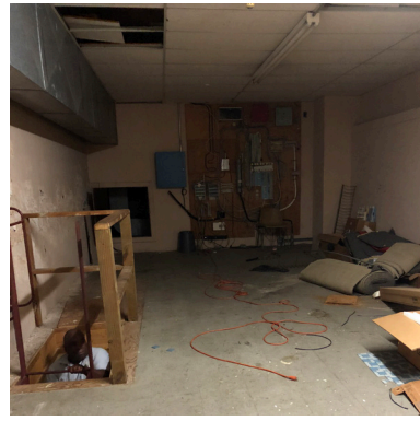
utility room | glen echo school
