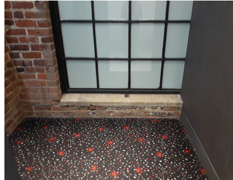
IMAGE IV: Opaque interior window joined with brick and cement wall. Flooring appears to be chip concrete. All windows of the building, save for two on the north wall, are sealed off from the inside.
