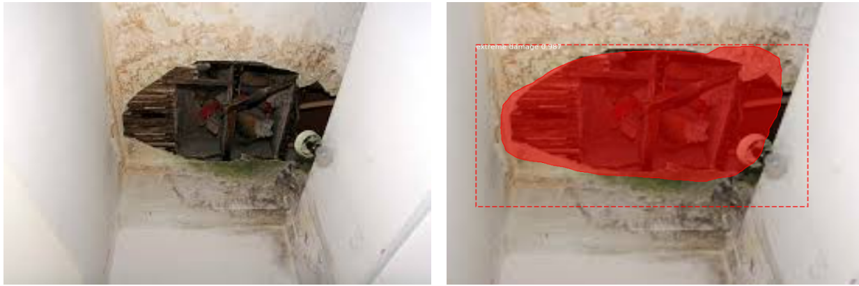
Figure 5.6: Extreme Ceiling Damage using Mask-RCNN Showing Instance Segmentation.
