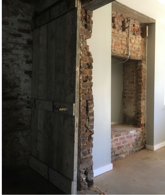
Original carriage house threshold and filled window on west wall adjacent to market
