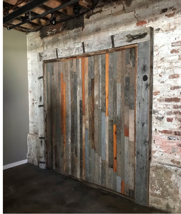
Filled door on west wall adjacent to market
