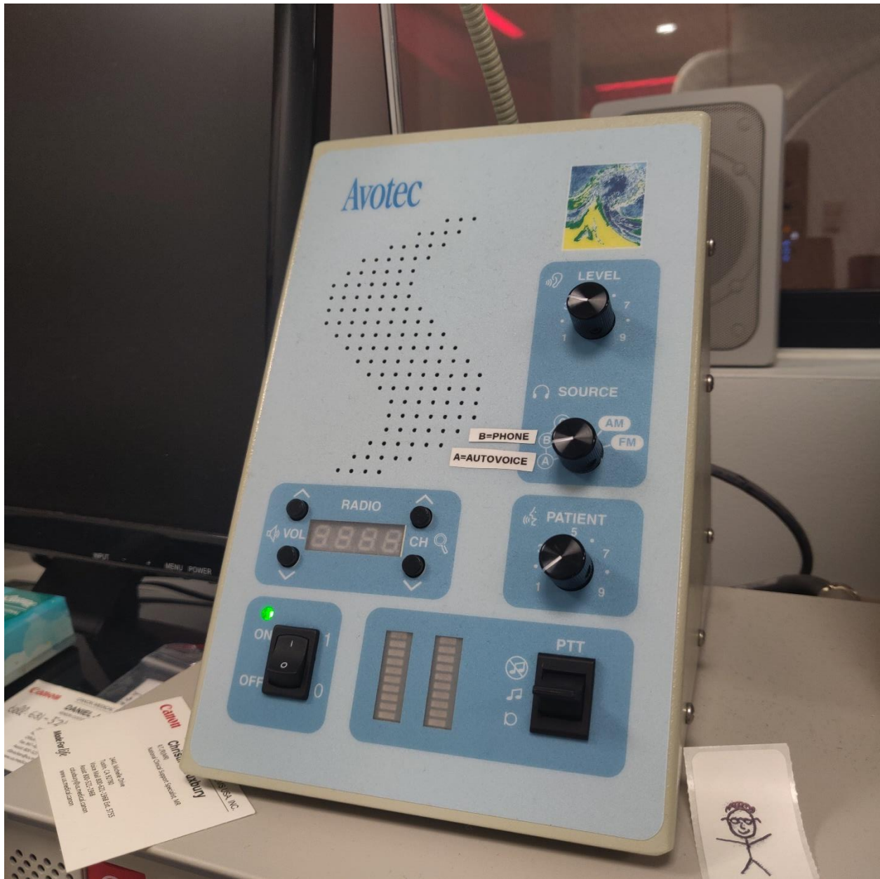
Figure 9: Photo of the patient intercom system.
