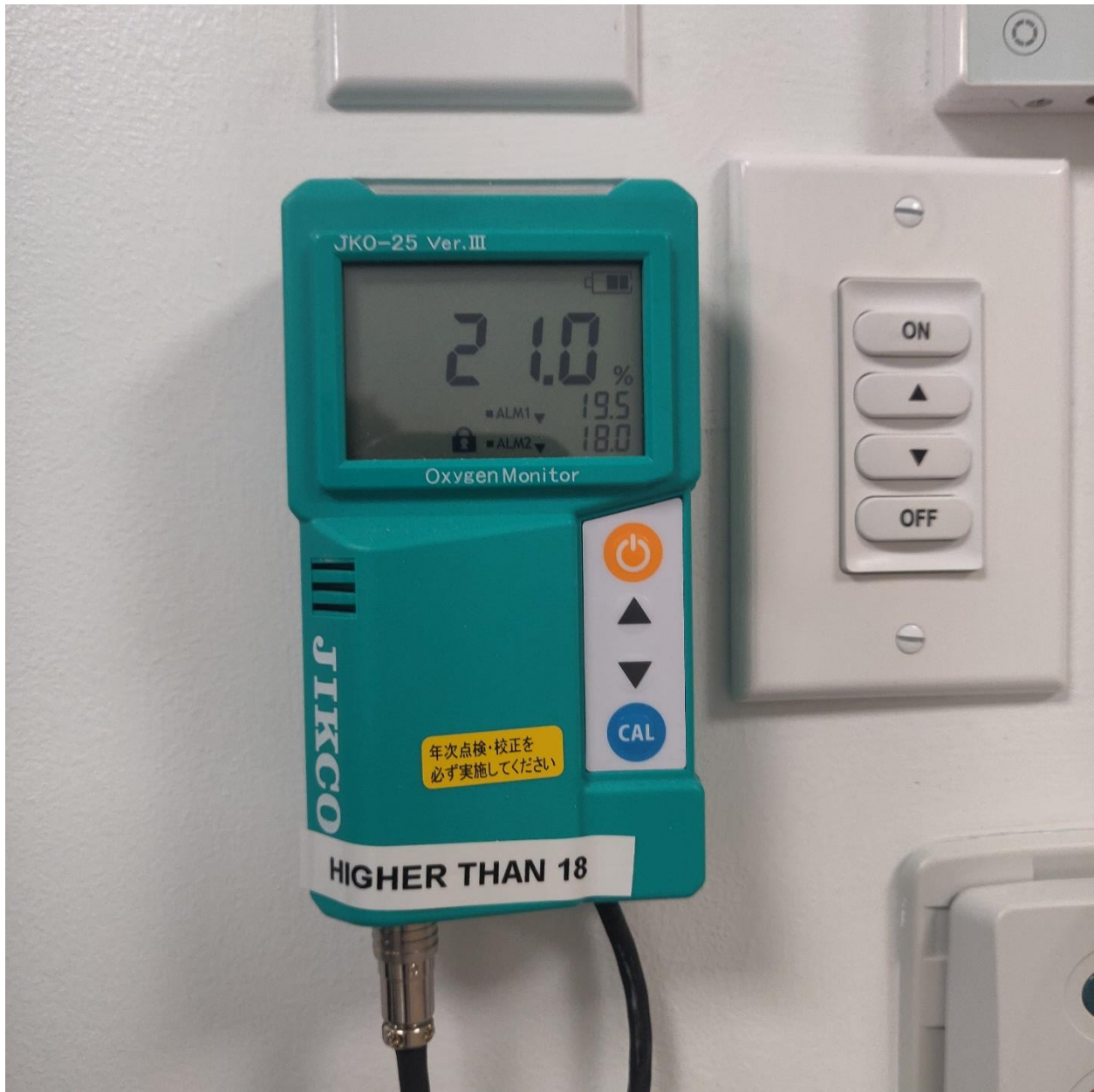
Figure 8: Photo of the wall mounted oxygen monitor.
